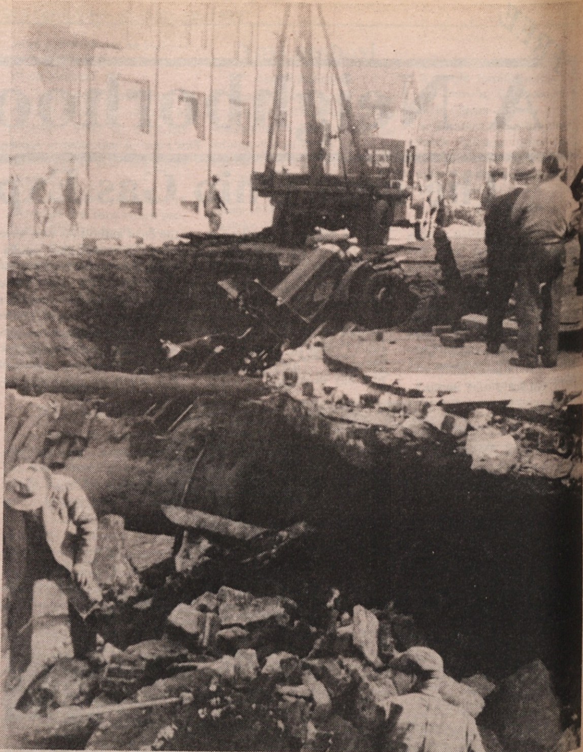
An underground gas explosion on E. 62 Street, just south of St. Clair caused this hole which trapped the fire engine shown in the top of the photo being pulled out.
