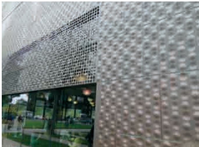
Slika 9: Perforirana in reliefno oblikovana bakrena pločevina na fasadi (Muzej mladih, San Francisco, Herzog & de Meuron 2005) [Foto: Zbašnik-Senegačnik]. Figure 9: Perforated and relief copper sheet metal on a façade (The de Young Museum, San Francisco, Herzog & de Meuron, 2005) [Photo: Zbašnik-Senegačnik].
