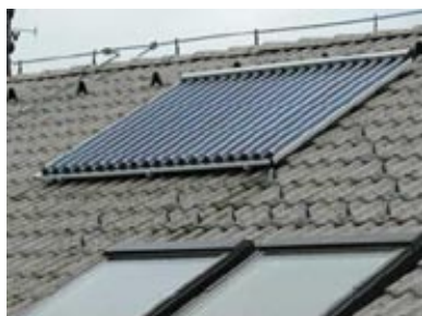
Figure 8: Fixed solar collectors
