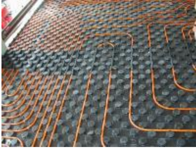
Figure 13: Underfloor heating system
