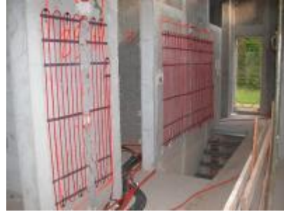
Figure 14: Wall heating system
