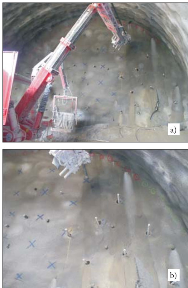
Figure 3. Example of face reinforcement in a shallow tunnel using longitudinal fibreglass pipes (Avigliana Tunnel, Turin, Italy): a) view of the face during the drilling stage; b) details of the reinforcement intervention with the pipes already in place.
