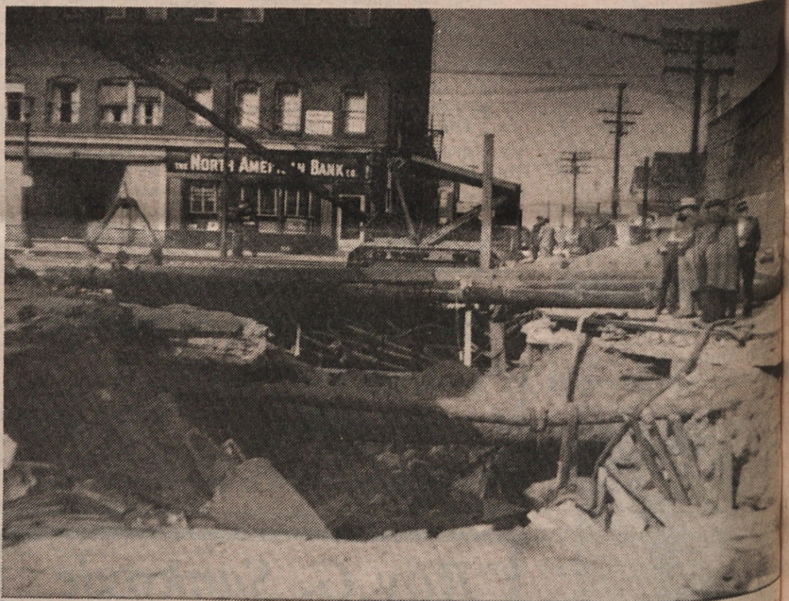
Scene at E. 62 and St. Clair after East Ohio Gas Explosion on Oct. 20, 1944 caused the cave-in of the street. The Novak Confectionery Building was weakened structurally and was razed. Joe and his wife, the late Mary (nee Milavec) reopened a card shop two stores to the west. The Novaks retired in 1972 after 52 years in business on St. Clair Ave.
