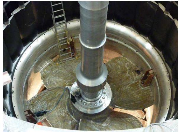
HE Krško – Rotor kaplanove turbine 1. agregata.
