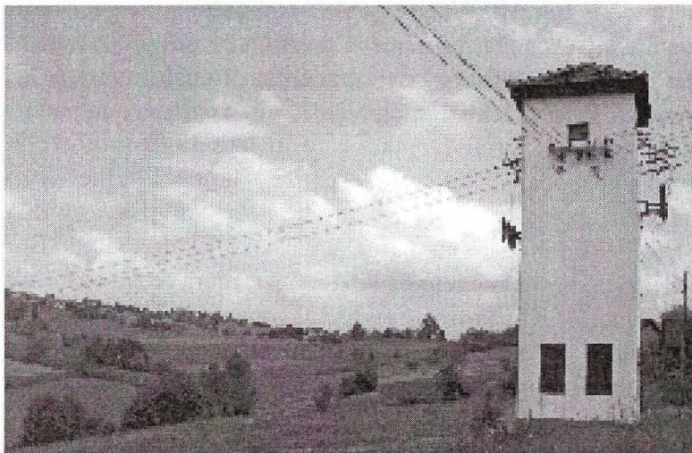
El. trafo v Jastrebcih danes
