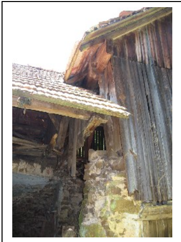
Podrta stena in obok stare kleti
