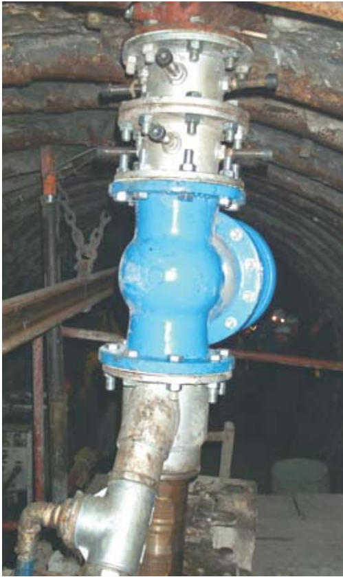
Figure 4. A flange of the conductor pipe, brakes, a valve, and a swivel pipe Slika 4. Prirobnica uvodne kolone, zavore, zaporni zasun in izlivka
