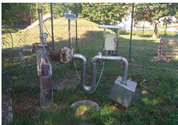
Figure 4: Wellhead of thermomineral water well RT-1/92 with a monitoring system.
