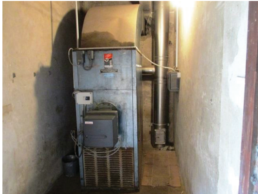
Figure 3: Boiler room with ELFO boiler
