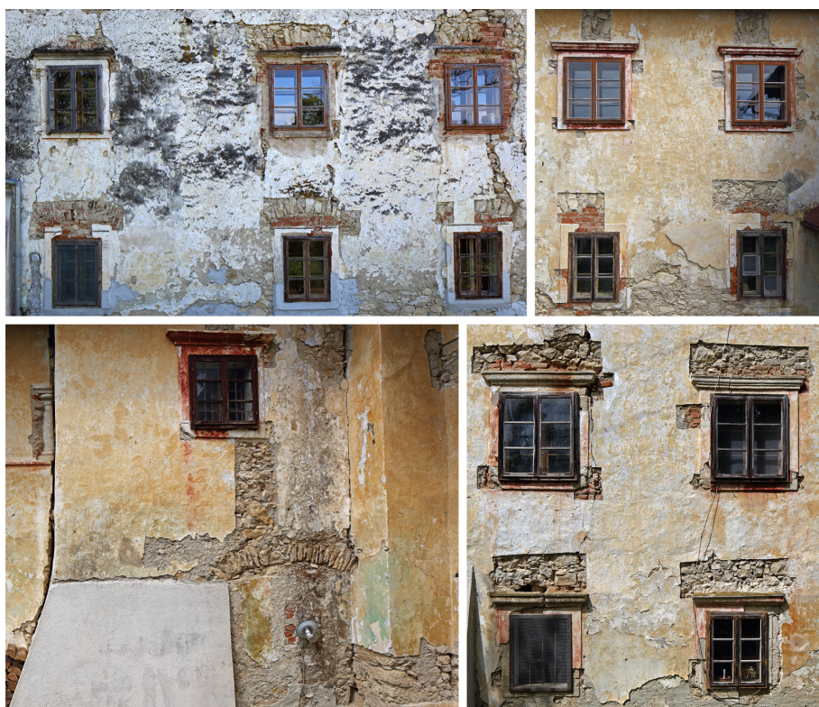
Fig. 1: Zagorska Sela, Poklek Manor, window axes of western façade (above left); western section of southern façade (above right); portion of transversal protrusion and eastern section of southern façade (below left; southern portion of eastern façade (below right), photo: J. Rasol, 2016.
