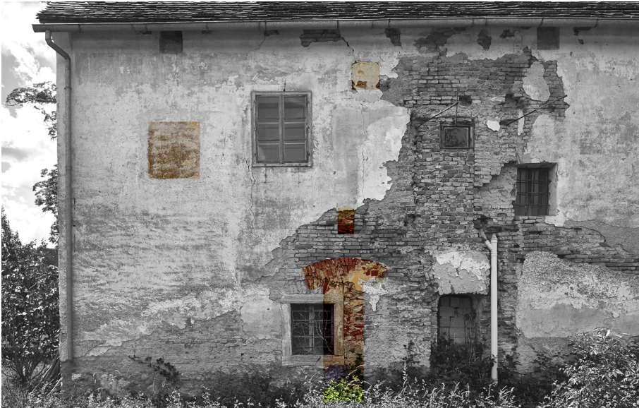
Fig. 6: Borkovec, southern part of eastern façade, photo: J. Rasol, 2016; print: R. Mavar.
