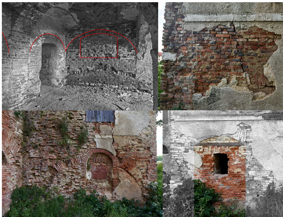
Fig. 5: Poznanovec, Sermage Mansion, southwestern portion of the rectangular ground-floor room believed to be a part of the original core (above left); built-in window and traces of an earlier plaster layer in the ground-floor of the northern part of the western façade (above right); ground-floor of eastern façade of western projection (below left); part of southern façade of western projection (below right), photo: J. Rasol, 2016.; print: R. Mavar, 2016.
