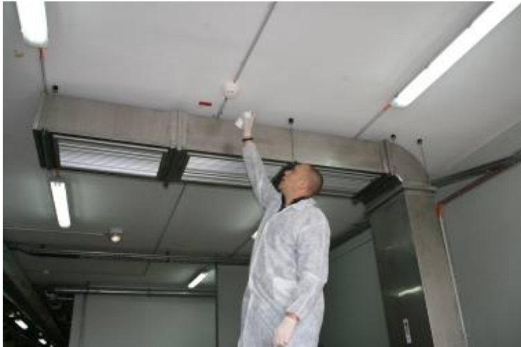
Figure 12: A function test of smoke detectors in CSRW
