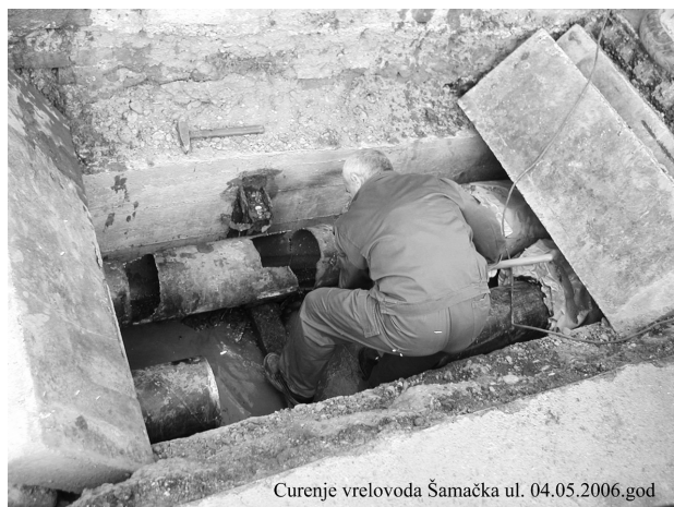
Figure 1: Leaking of hot-water pipes during use
