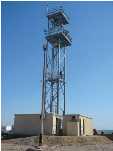
Fig. 2. Pylon and optronic sensors.
