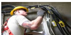
Identify faulty cables at manhole with other cables still carrying traffic
