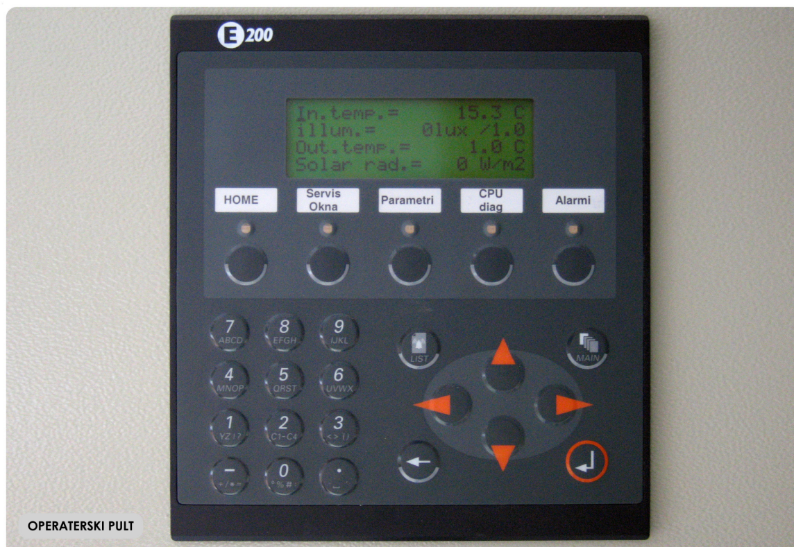
Slika 3.10: Pogled na operatorski pult MAC/MTA E200. Fig. 3.10: Operational platform MAC/MTA E200.
