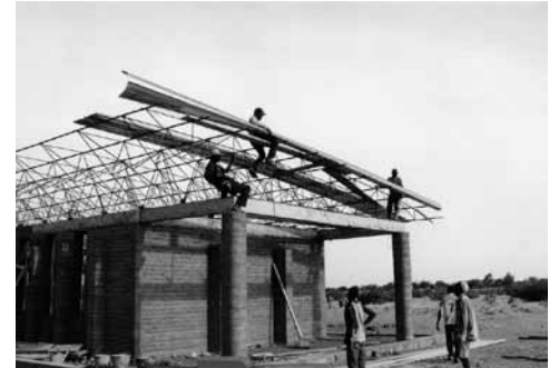
Osnovna šola v vasi Gando, 2001, med gradnjo strehe. Elementary School in Gando, 2001, the construction of the roof.
