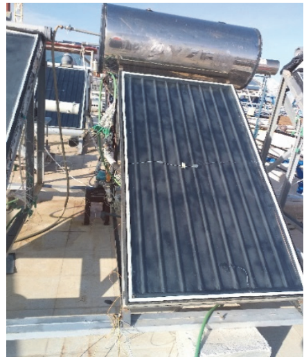
Solar water flat plate solar collector
