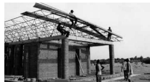
Osnovna šola v vasi Gando, 2001, med gradnjo strehe. Elementary School in Gando, 2001, the construction of the roof.
