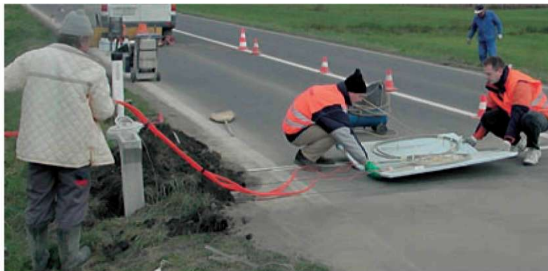
Fig 1: Live road installation of an experimental fibre optic axle detector near Sp. Polskava.
