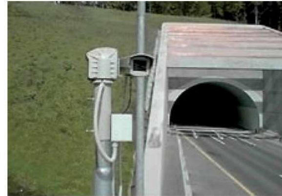
Optical Communications Traffic Control Systems.
